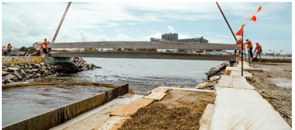
Lowering of the bridge structure was meticulously planned and executed by the project team.
