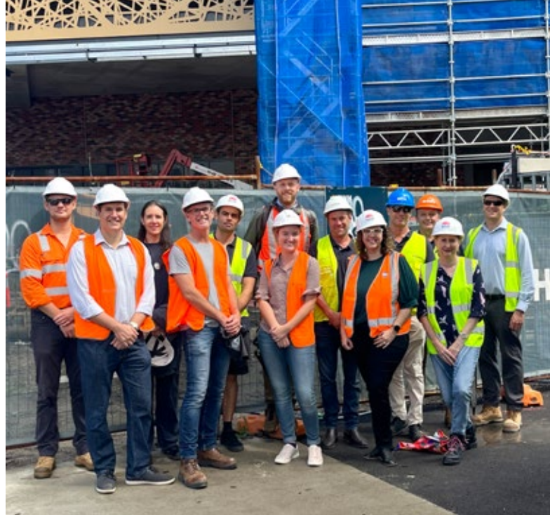
Thanks to GWH Build for taking HCCDC team members on a site tour of the soon to be completed building and public space.
